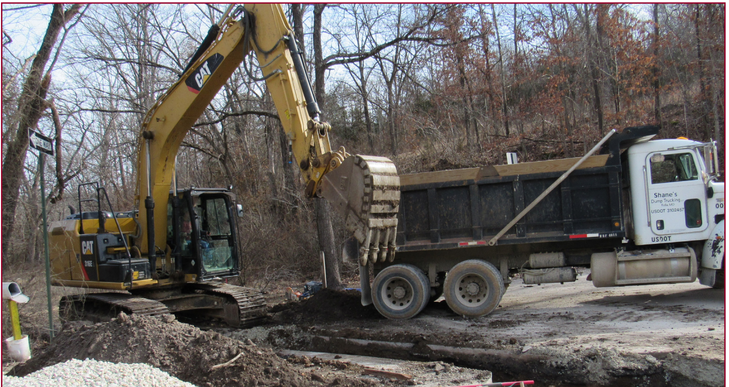
Crews begin work on the Newburg Community Development Block Grant to make significant improvements to the water system including a new storage tank, well house and distribution lines in February 2024.
